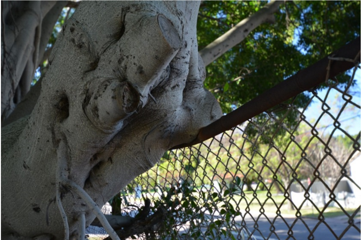
FIGURE 9: BRANCHES REMOVED TO TREE 3 TO RELIEVE PRESSURE ON BOUNDARY FENCE AND PREVENT FURTHER BUCKLING.
